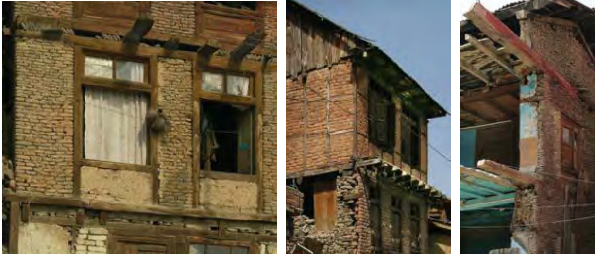
3.6.1 a, b & c Photographs showing construction details of taq buildings. The one on the far left shows the front wall perpendicular to the joists in a taq building, showing how the joists are sandwiched between the timber bands. The second shows how the secure connection of the joists to the front wall bridged the earthquake-collapsed rubble-stone side wall. The third show a taq building partly demolished, exposing the timber lacing in the wall parallel to the joists.
