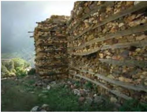
3.3c Early 20th-century fort in Besham, Pakistan after the 2005 earthquake, showing how the collapse of this dry-laid rubble stone wall was prevented by the timber lacing. This demonstrates the effectiveness of the timber tie beams (bhatari) in holding the earthquake-damaged rubble stone wall together.
