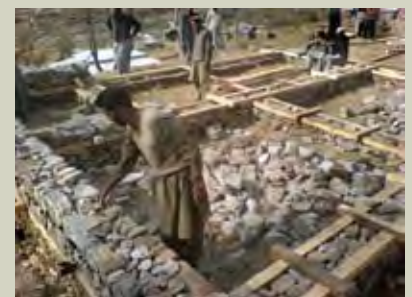
3.3e, f & g Views of a training workshop on bhatar construction for local masons in Battagram, Pakistan, in spring and summer 2007, prepared by the French Red Cross with Architectes et Développement. Photos by the French Red Cross.
