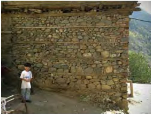
3.3b Traditional bhatar construction in the Swatt Valley town of Behrain used to stabilize a rounded random rubble stone wall construction which otherwise is extremely at risk in earthquakes.
