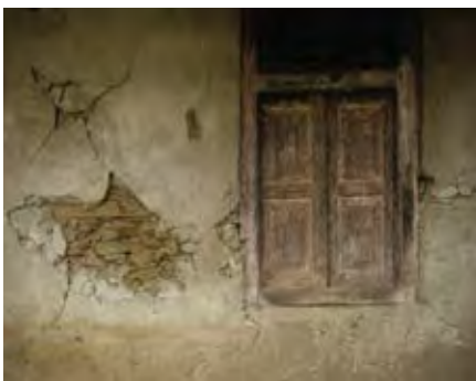
3.2b The side of a timber-laced masonry building near Uri after the 2005 earthquake: The quake caused the cracking of the modern rigid cement plaster from the otherwise non-destructive shifting of the underlying timber-tied masonry.
