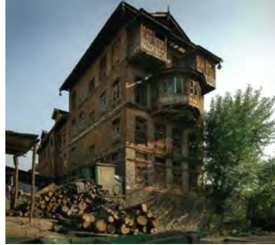
3.6.3a A once splendid five-storey house of taq construction along side the Rainawari canal, Srinagar. These large houses in the Rainawari area are constructed on the very soft soils of what was once the middle of Dal Lake. The timber lacing is essential to their stability, and their age and durability demonstrates that multi-storey buildings of masonry and timber can be safely built.
