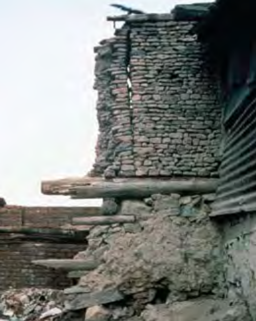
1.1d House under demolition showing how the masonry wall of taq is subdivided into panels where the light shows through between the wall panel and the half-demolished pier.
