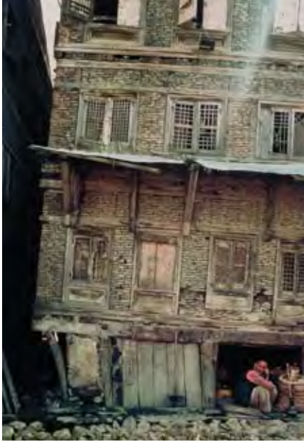
1.1a 18th- or early 19th-century canal shop house alongside what was once the Mar Canal in Srinagar. This building survived the 1885 earthquake. The timber lacing has held this structure together despite extensive differential settlement. Note that the windows are not lined up vertically: this feature would not be structurally possible had the walls not been reinforced with timbers.
