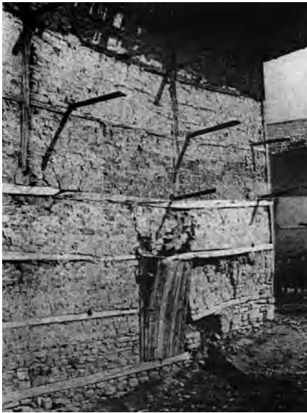
3.2a Photo by Turkish Professor Alkut Aytun showing a two-storey brick house with timber bond beams spanning the ground rupture from the 1970 Gediz earthquake in western Turkey. In the caption to this image, he observes that this shows the effectiveness of timber bond beams for both fired or unfired brick masonry (Aytun, 1981).
