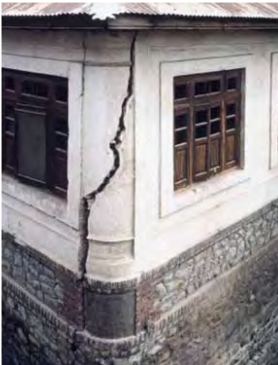
1.1g Photograph taken in the 1980s in Srinagar of an unreinforced masonry building without timber lacing, showing how soil subsidence is causing the structure to come apart.
