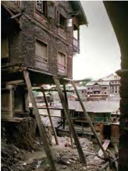
1.1b Taq building on the bank of the River Jhelum. The fact that this bearing wall masonry structure can be held up on three poles is a testament to the effectiveness of the timber lacing. The shoring poles are supporting the structure under the three main beams that support the joists, two of which are embedded in the front and back masonry walls.
