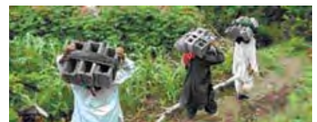
3.3k Cement blocks for housing reconstruction being moved by footpath to a remote site. Source: ERR4, 2007.
