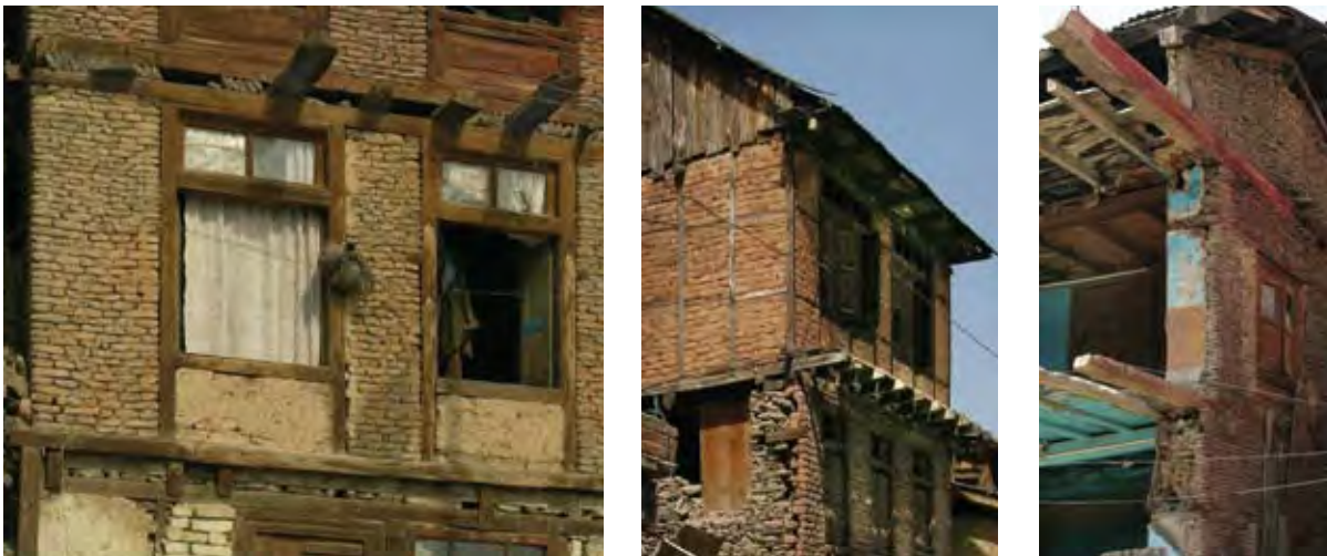
3.6.1 a, b & c Photographs showing construction details of taq buildings. The one on the far left shows the front wall perpendicular to the joists in a taq building, showing how the joists are sandwiched between the timber bands. The second shows how the secure connection of the joists to the front wall bridged the earthquake-collapsed rubble-stone side wall. The third show a taq building partly demolished, exposing the timber lacing in the wall parallel to the joists.
