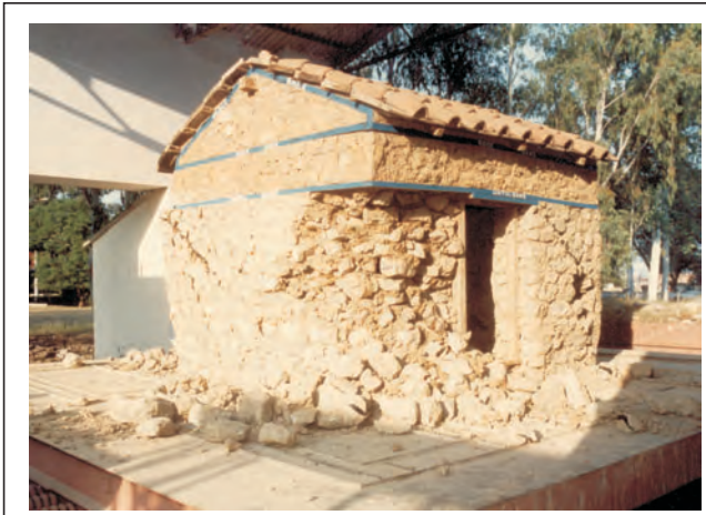
Fig. 7 Partial collapse below lintel band
