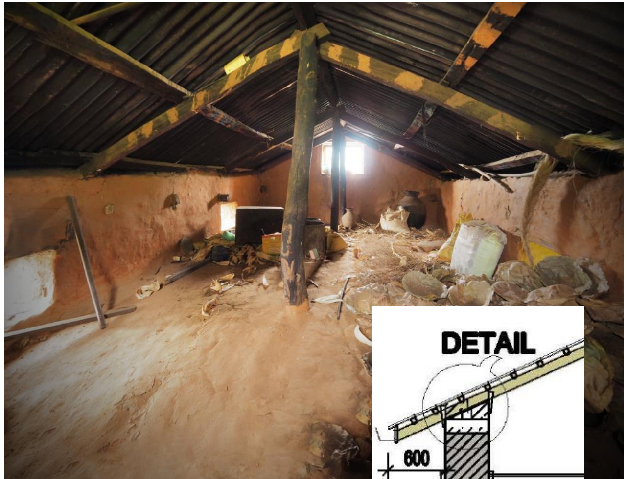
Above: Interior of attic of Nepal Family house in Mankhu showing the masonry walls extending up above the attic floor – which is also shown on the right in the DUDBC design for “Stone Masonry with Mud Mortar SMM-1.1. The Nepal Family house suffered very little damage in the earthquake.
